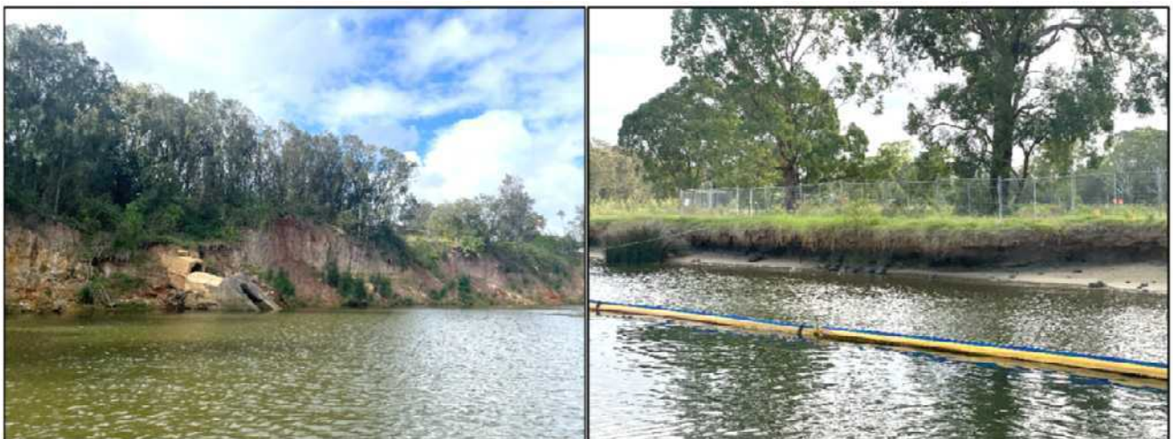
Plate 6 Examples of Extreme erosion severity in the study area, from left to right: upper Georges River Reach 264; mid Georges River Reach 250.
