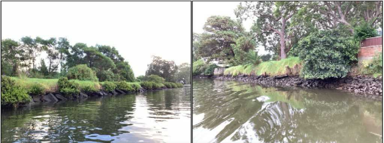
Plate 18 Examples of inappropriate bank protection works in the Georges River estuary, from left to right: dumped concrete slabs on the mid Georges River Reach 9; and building rubble used for bank protection in the upper Georges River Reach 35.
