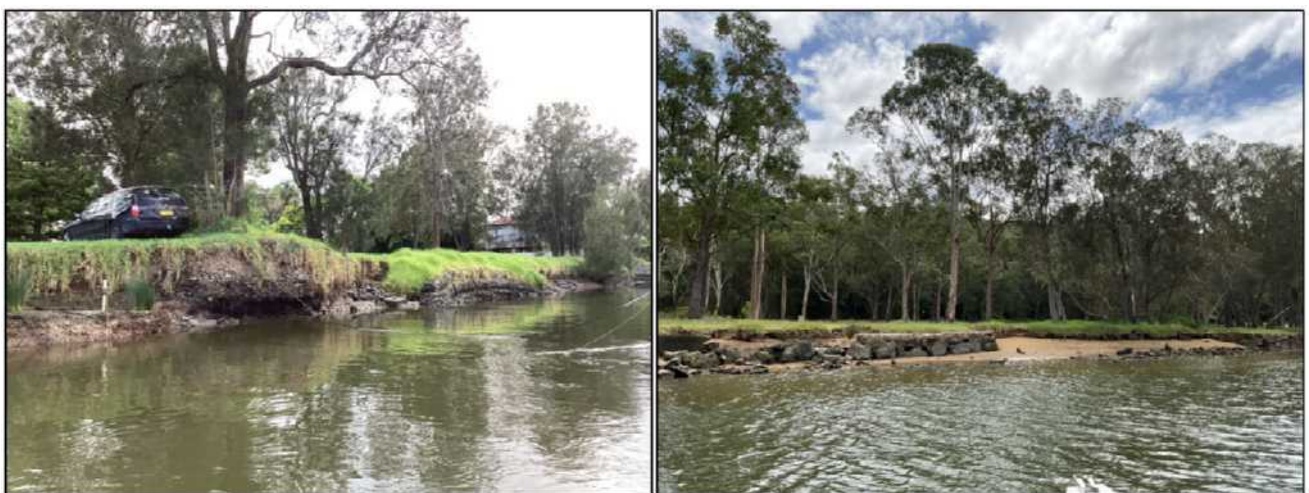
Plate 17 Examples of ineffective bank protection works in the Georges River estuary, from left to right: failed gabion structures on the upper Georges River Reach 26; and failed rock works with concrete capping on the mid Georges River Reach 394.
